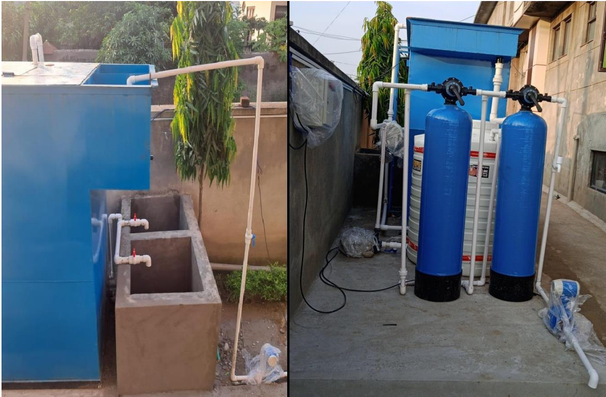
15 KLD STP/ETP Plant
